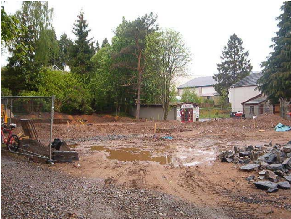
Fig 4. Current construction site for bus lay-by and landscaping on village green, application site behind trees.
